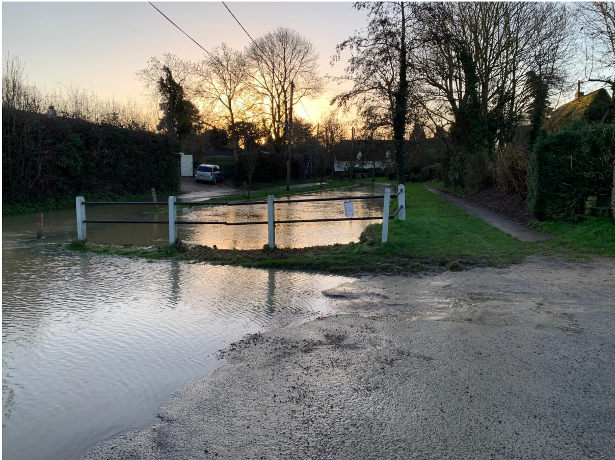
Flooding to Brook Street at the upper culvert entrance of the Elsworth Brook.
